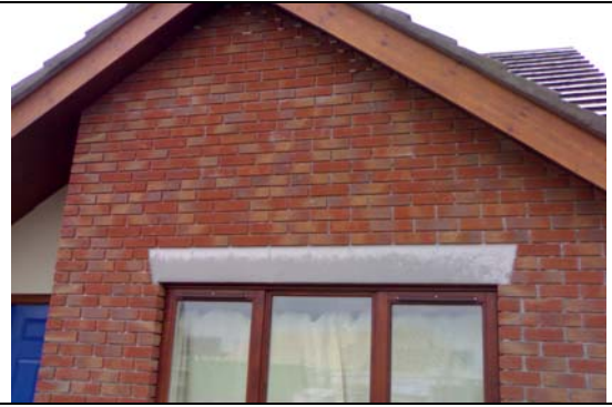
Brick slips are 7429HL from the Celina Klinker range from Padipa Ltd. Ardex adhesive used. All work undertaken by contractor.
